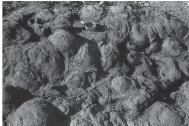
Fig.6.4 : Exfoliation (Flacking) and granular disintegration
